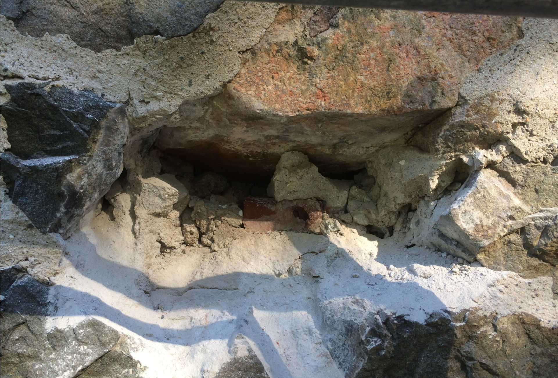
View of exploratory opening to expose make-up of structural wall at Tower B
