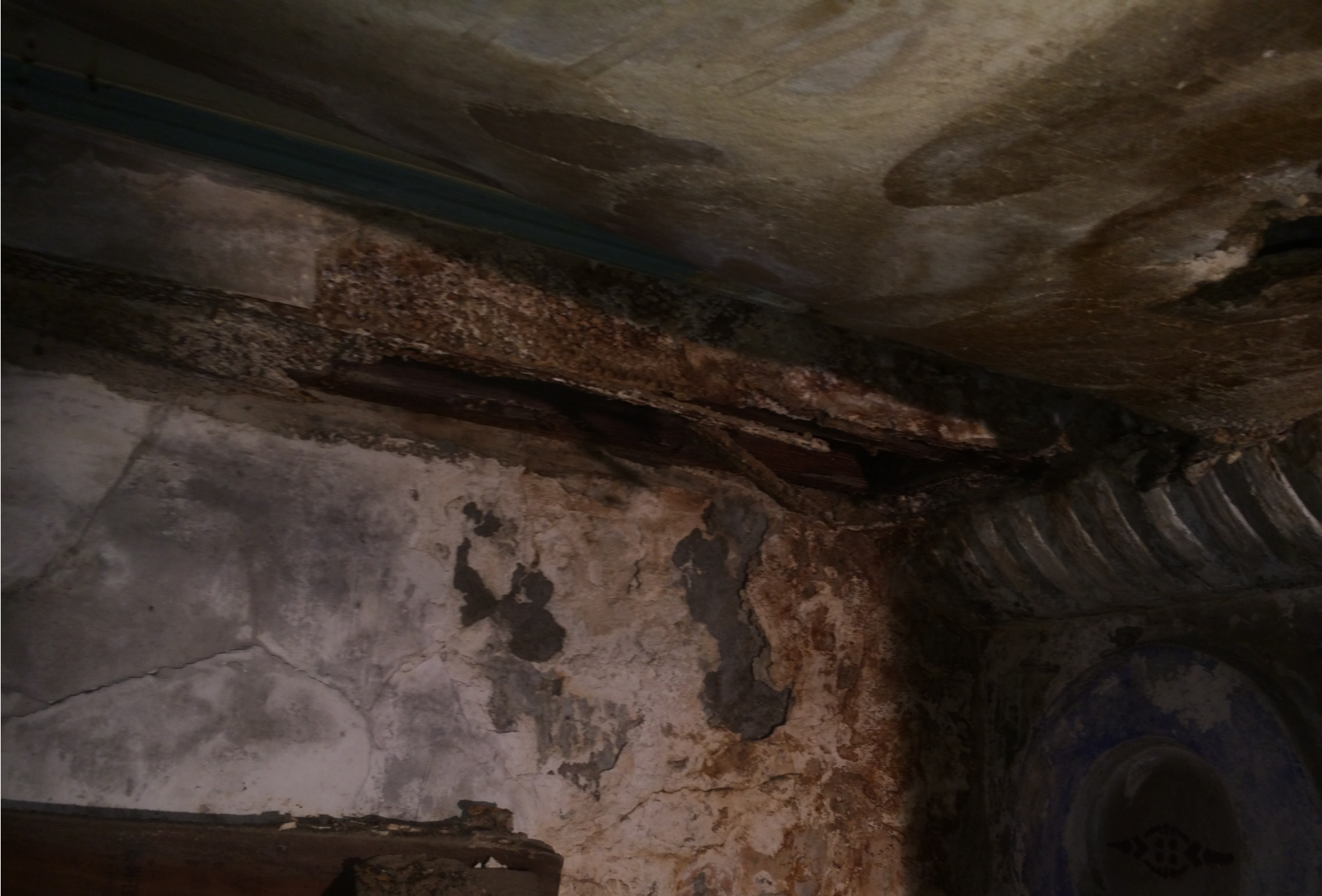
View of moisture damage on plaster and corroded metal structure in Tower A abandoned stairway
