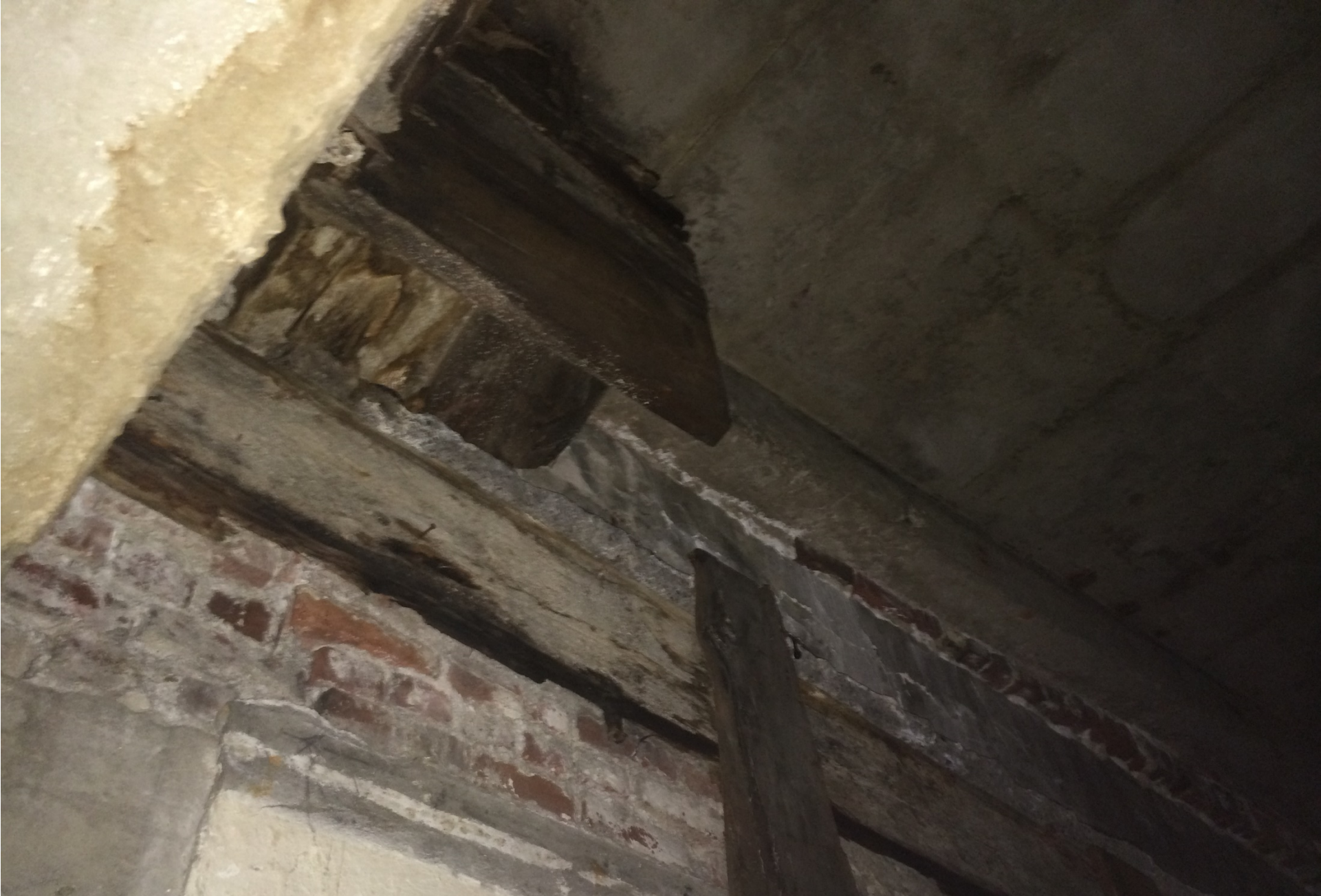
View of moisture staining of wood structure in Tower C
