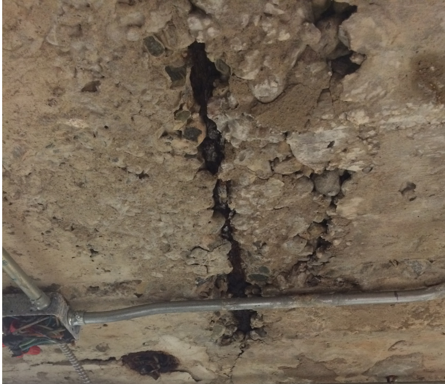
View of the cracks and voids in the underside of the concrete slab at Tower C entry.
