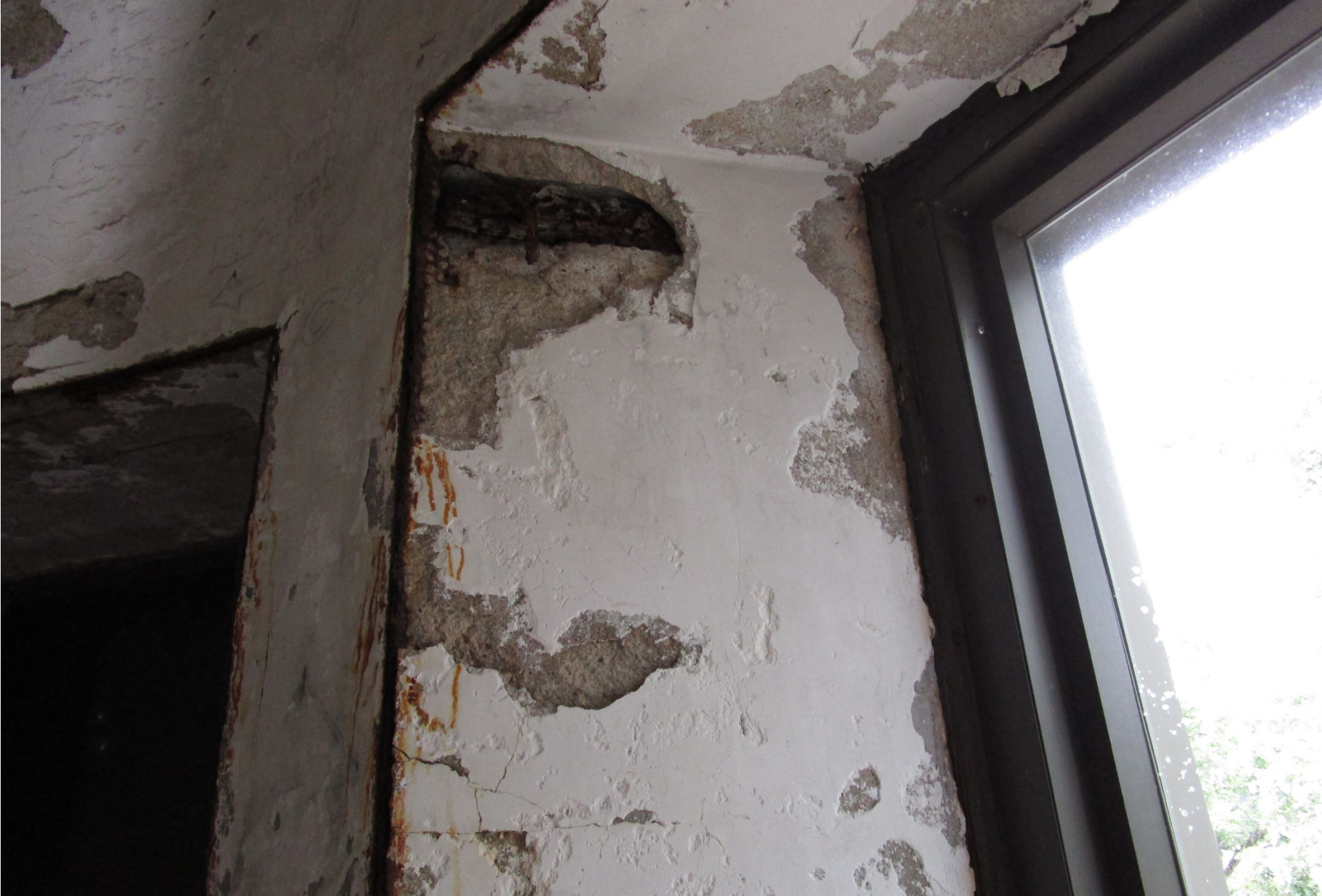
View of plaster damage and corrosion at Tower A abandoned stairway
