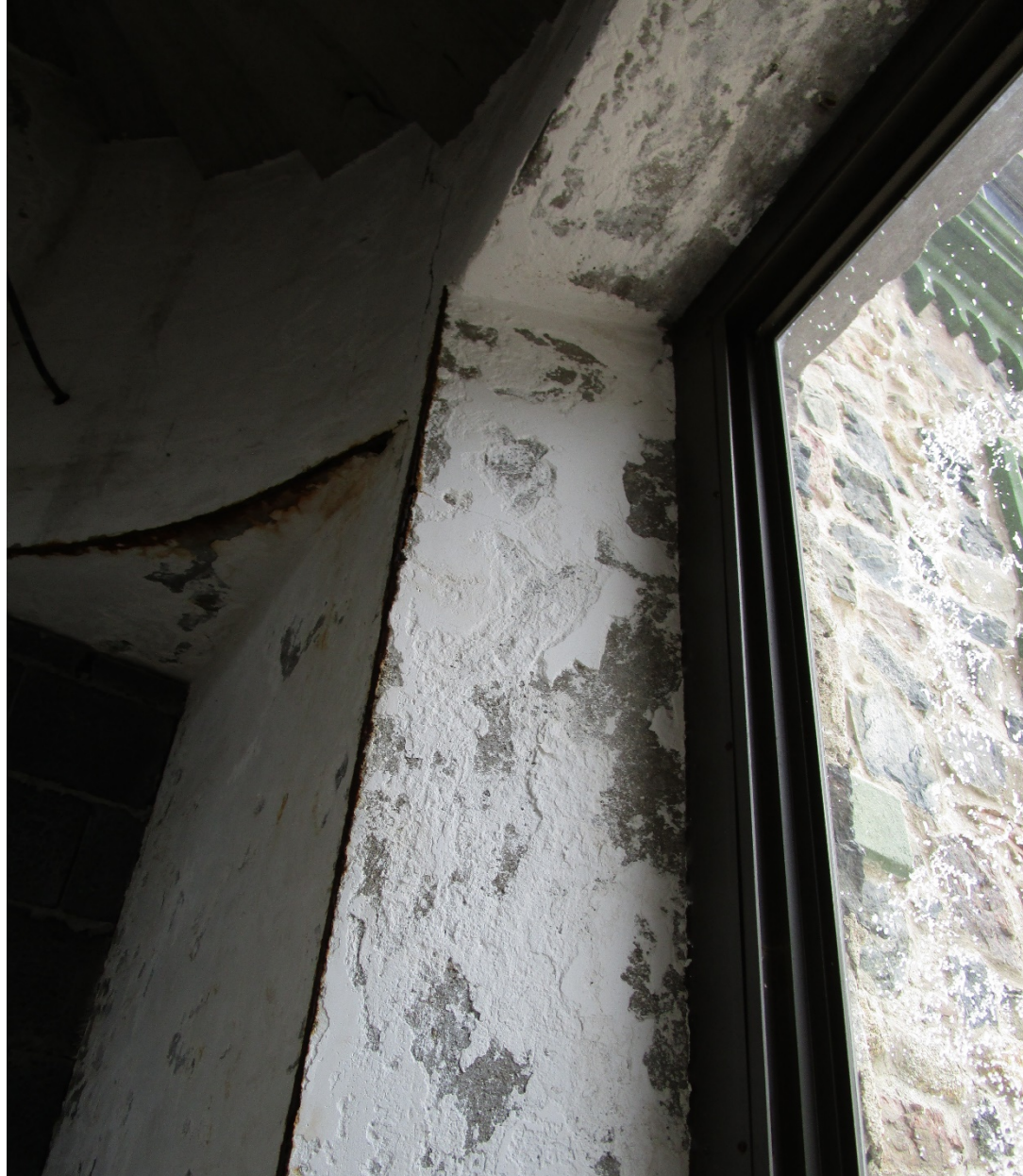
View of plaster damage and corrosion at Tower A abandoned stairway
