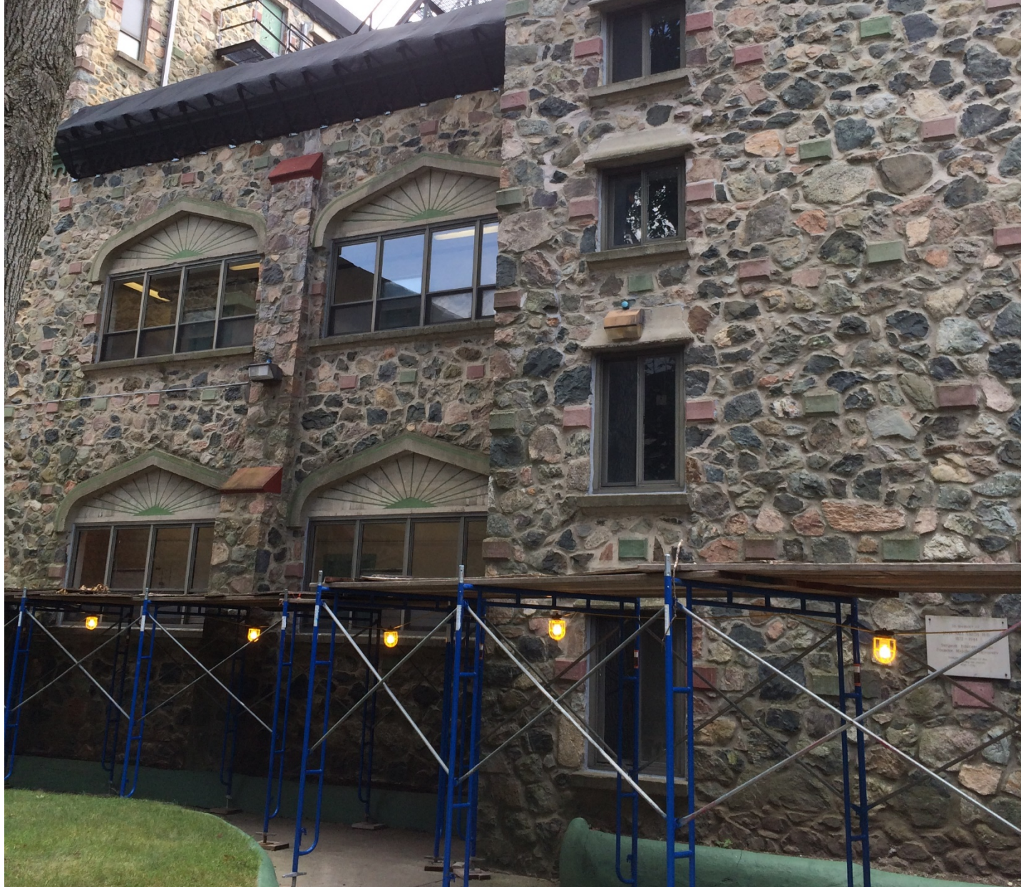
View of protective scaffolding at walkways leading to Tower A and Tower B entries
