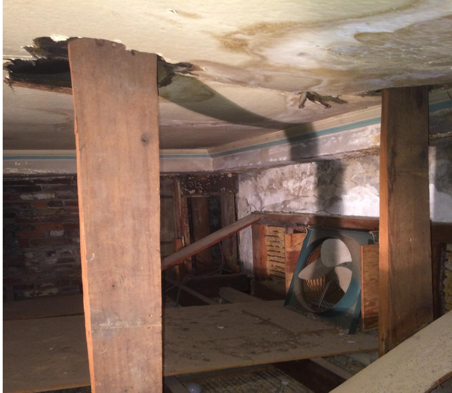
View of moisture staining on damaged plaster ceiling in Tower E
