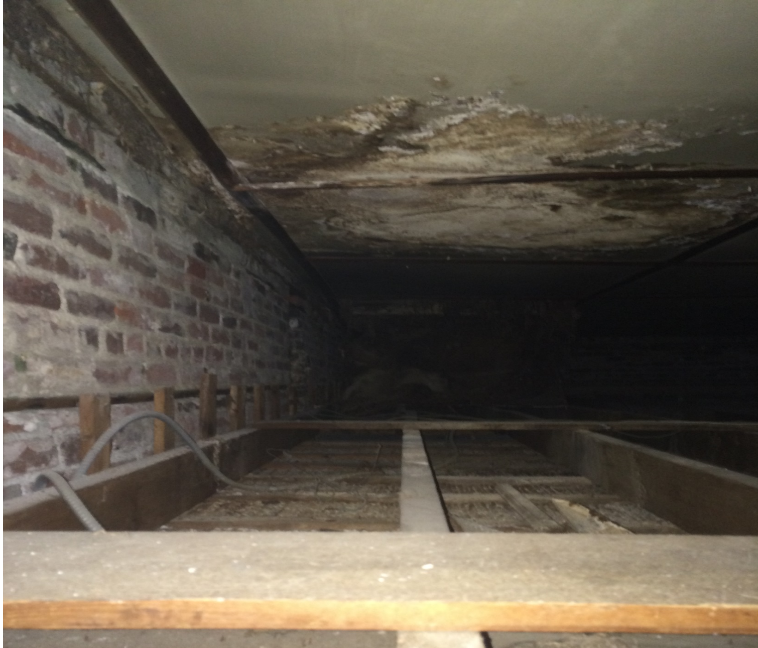
View of moisture staining in plaster ceiling in Tower A
