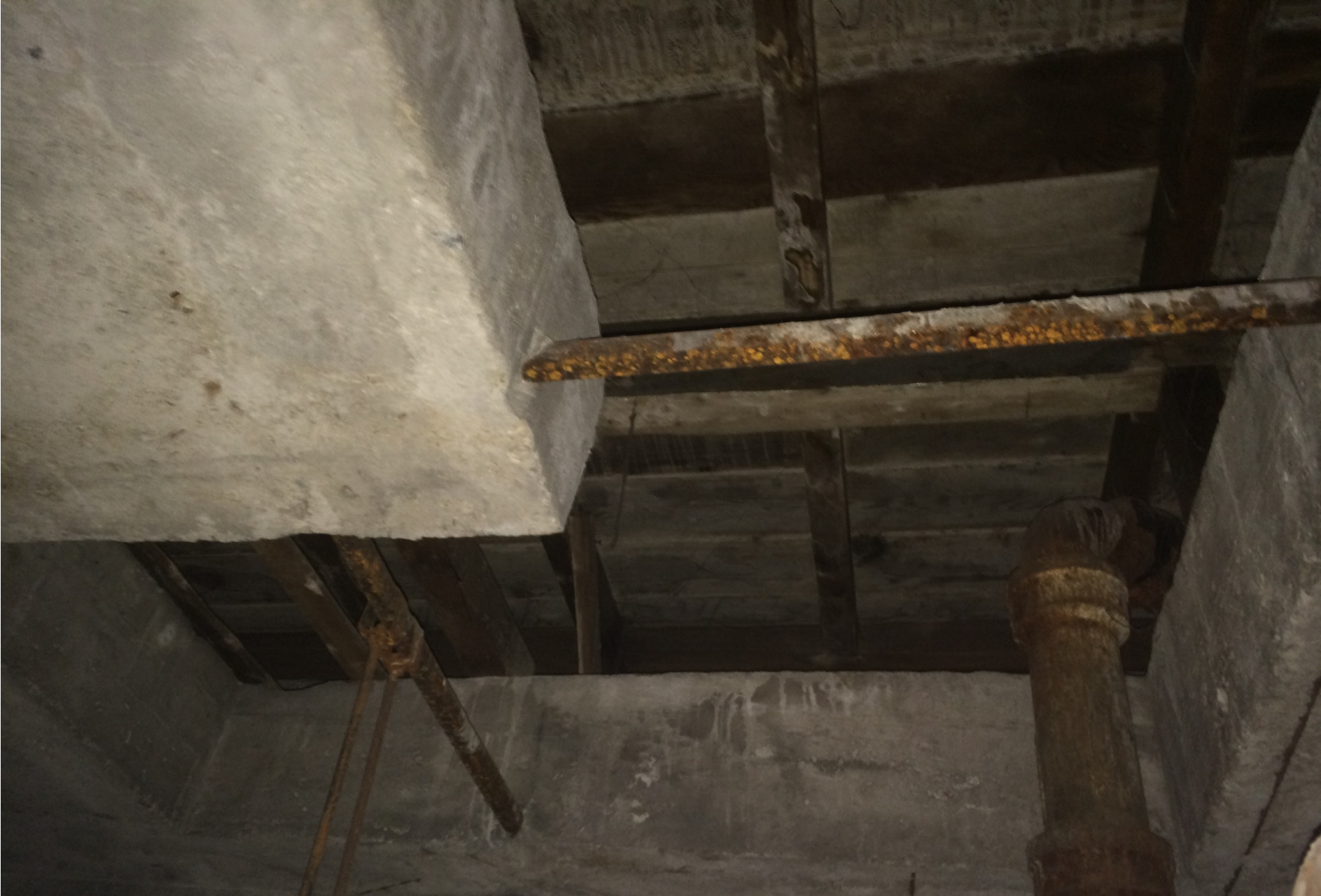
View of moisture staining on wood structure and corroded metal in Tower B
