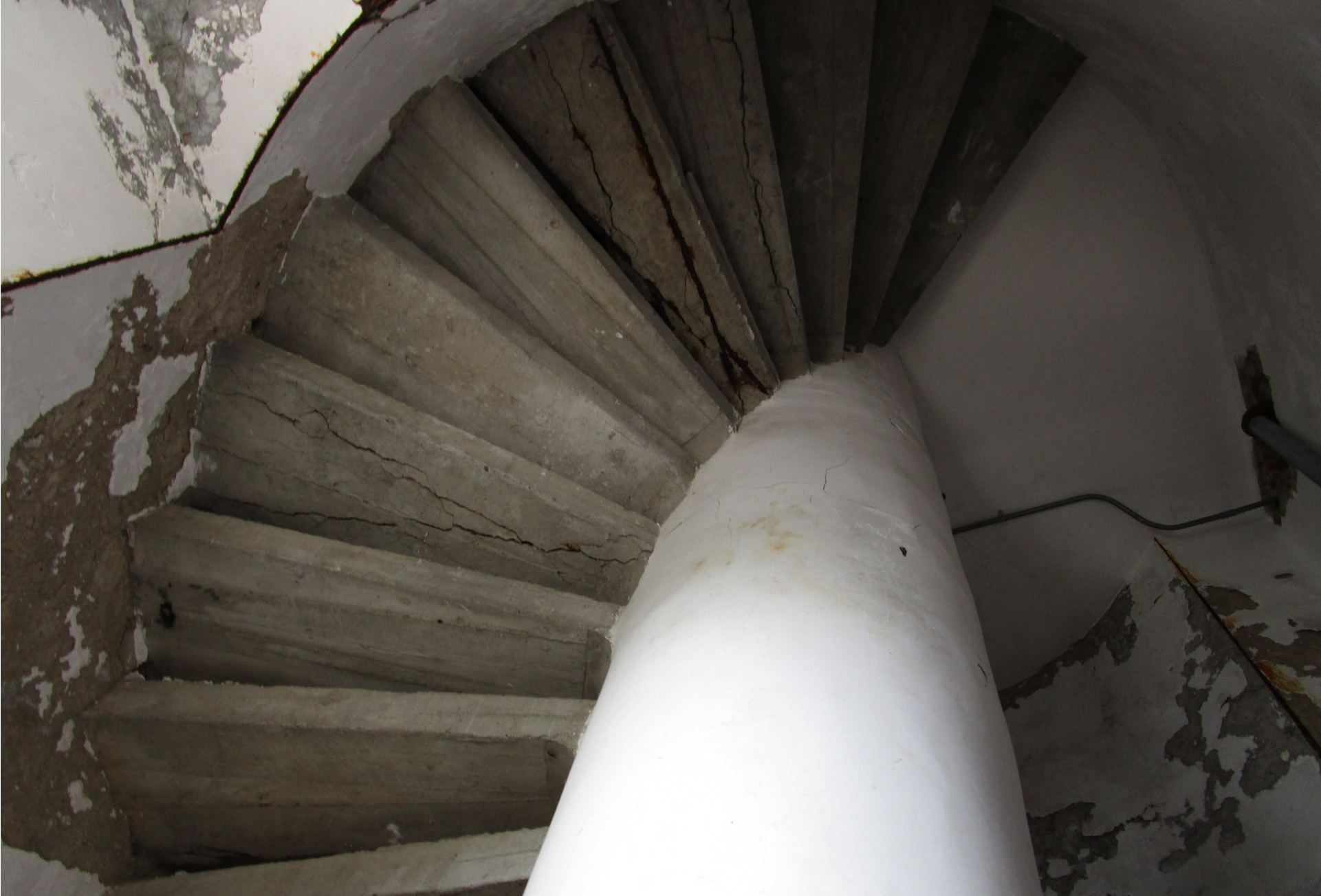
View of the cracked concrete and exposed reinforcing at Tower A abandoned stair
