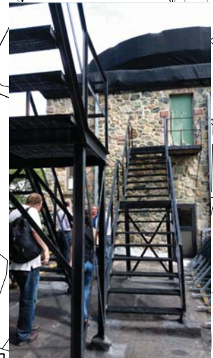
fire escapes used to provide egress between Towers A and B. Use of fire escape does not meet current code standards.
