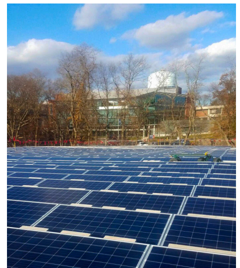
A new solar panel array was installed on the Library roof, doubling the amount of solar power generated on campus.
